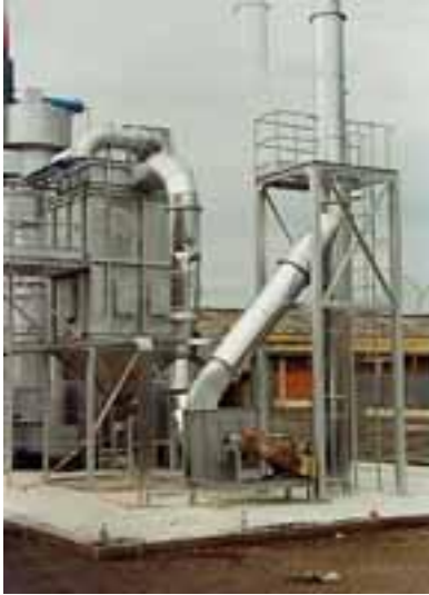
PSV FLUE GAS CLEANING SYSTEM WORKING
